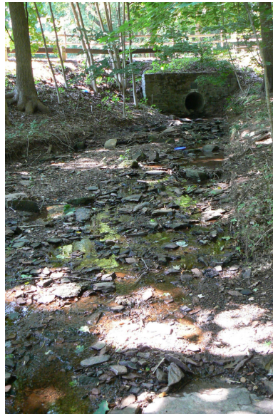
Sedimented streambed and streambank scour , Kunkel Park
